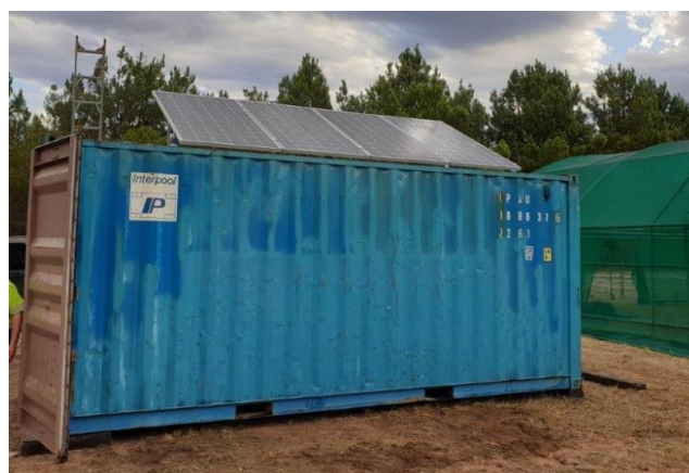
Figure 30: The complete on-site solar power system unit.
