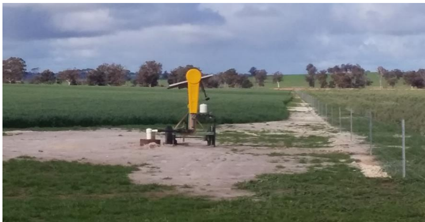
Figure 28: Yellow solar pump on the northern production bore.
