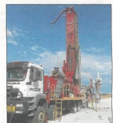
□ Two groundwater bores have been sunk to supply saline irrigation water to the bush foods horticultural growing system and simultaneously draw down problem groundwater levels affecting farmland.
